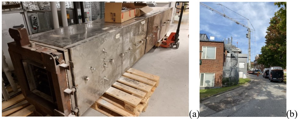
Figure 2. (a) The electric air pre-heater being instrumented and having necessary wiring fitted, before (b) reinstallation in the Lund high pressure-facility.
